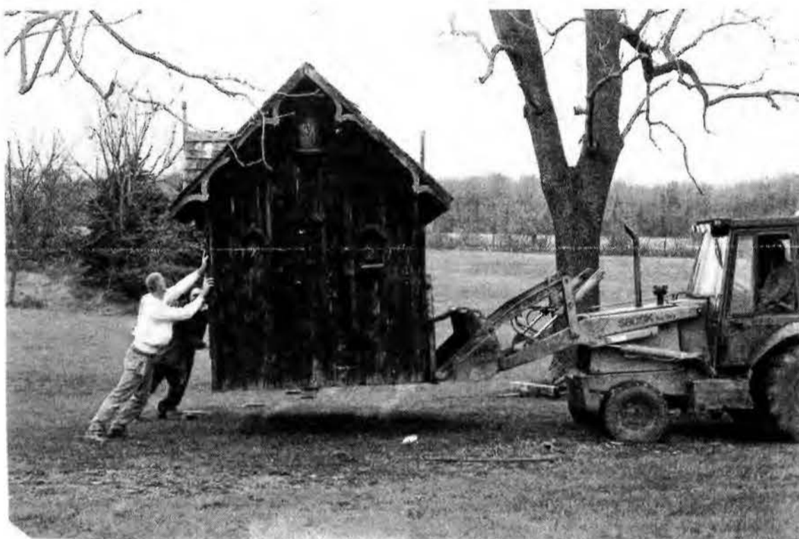
The Honey House is eased into its new location on the grounds of the Backus-Page House, December, 2006
